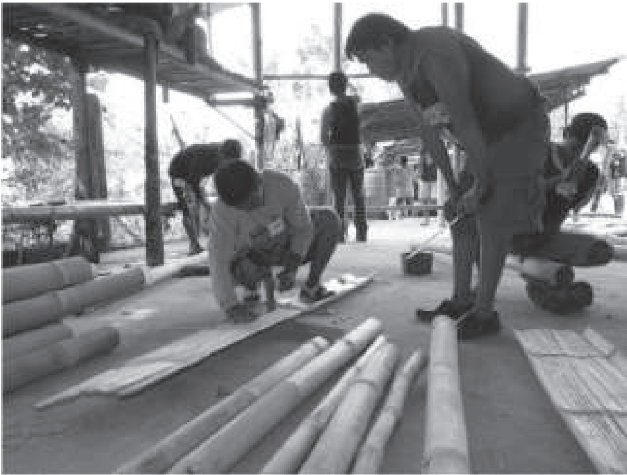
FIGURE 10.2 • Workers learned cutting, skinning, slatting, flattening (or “ tinadtad ”), and jointing of bamboo for construction
